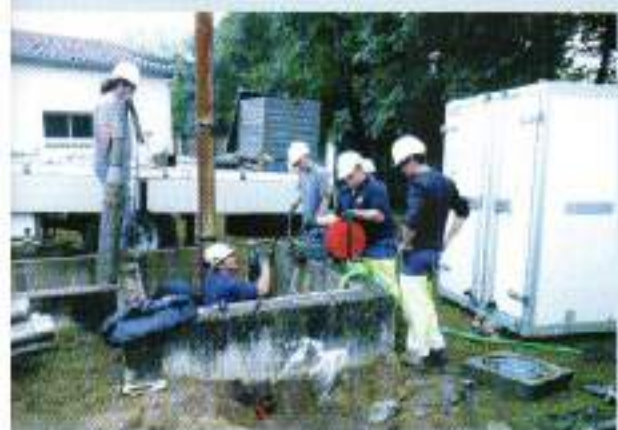
Station de pompage Route du Conte
